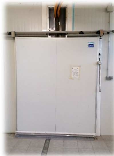
Refrigeration and freezing chamber.
